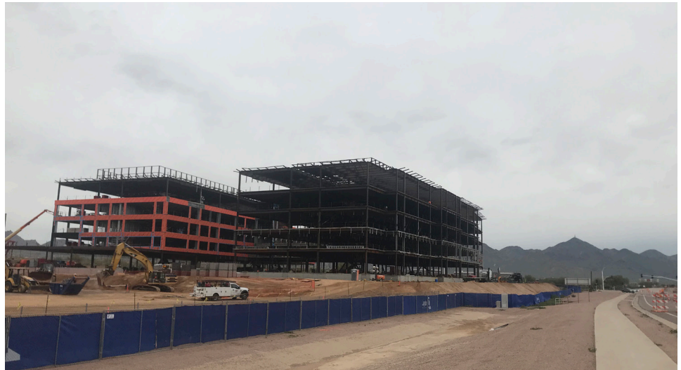
// Pictured Above: Nationwide Insurance building under construction at Hayden Road and Loop 101
